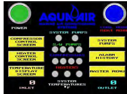
PLC / Touchscreen Chiller Controls
